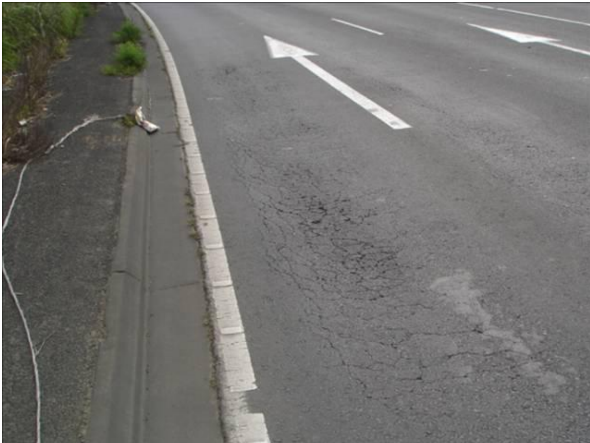
Figure 1 – Shear failure of basecourse aggregate.
