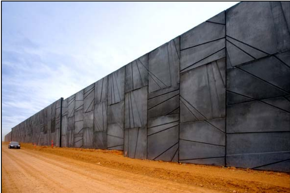
Noise Walls: Post + Panel
