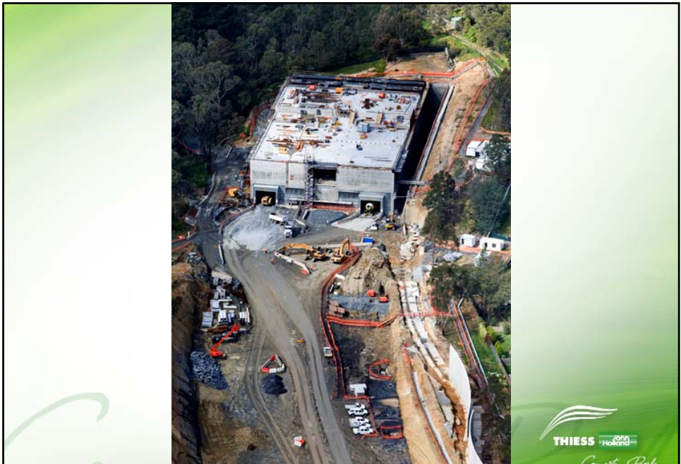
Tunnel – Ventilation Station
