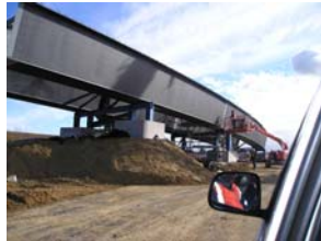
EastLink S/B Exit Loop over EastLink S/B Entry Ramp 240m, six span curved 2200mm deep steel trough
