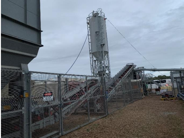
Koppens' Foam Bitumen plant
